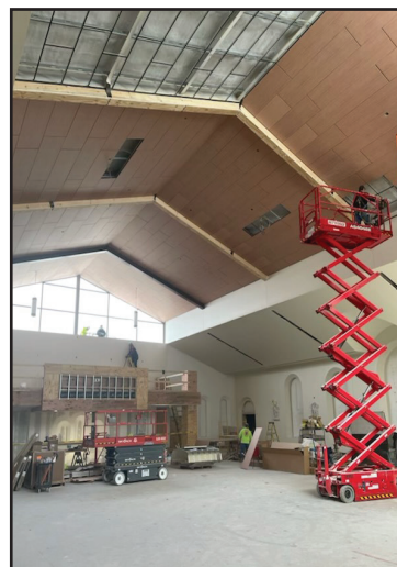
Old bleachers from the gym have been recycled for a new ceiling.
