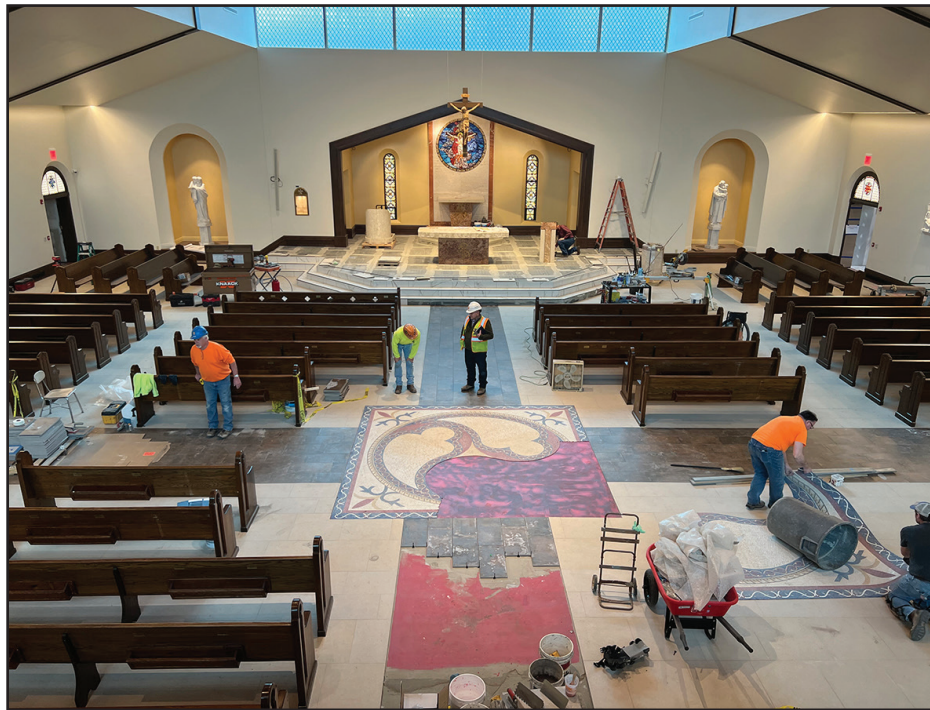
Workers from Sordoni Construction are close to completing renovations on the new worship space for Most Holy Trinity Parish in Cresco as seen on April 6, 2022.
