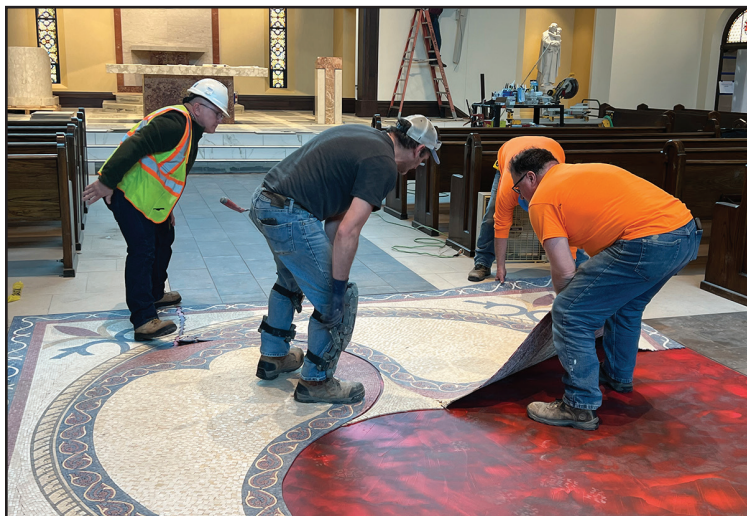
Workers put mosaic tile in place which will become the area for the baptismal font at Most Holy Trinity Parish.
