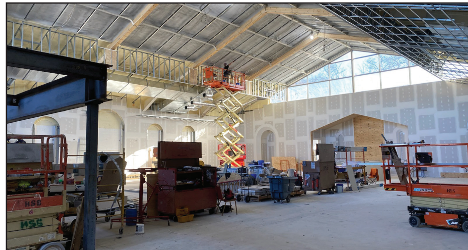
Below: Sordoni Construction has been working at the new worship site for Most Holy Trinity Parish in Cresco since September 2021.
