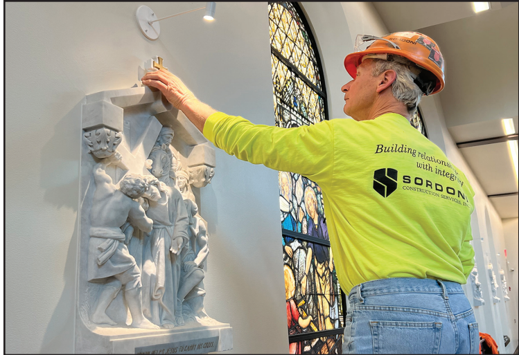
Ron Yanchak, a Sordoni Construction employee, glues a Cross in place on the top of one of the Stations of the Cross.
