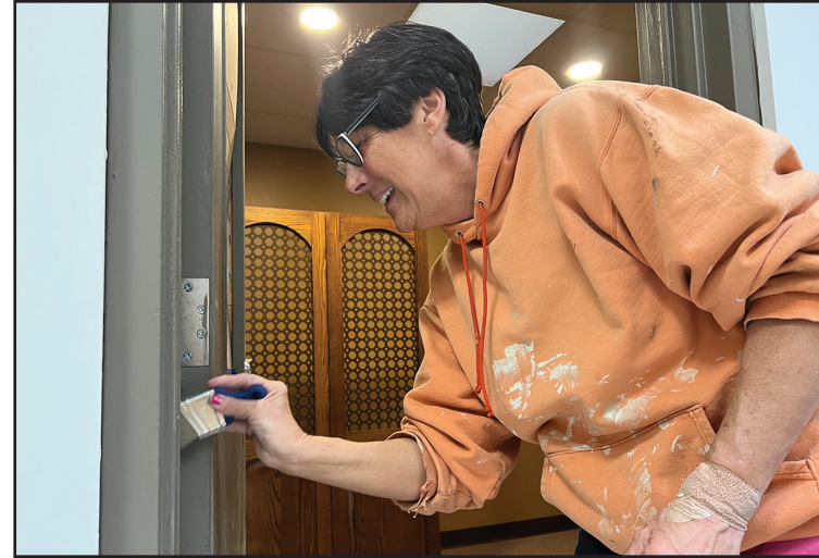
Cheryl Lynott of Paradise Township is one of many parishioners who is helping to renovate the new worship space for Most Holy Trinity Parish.
