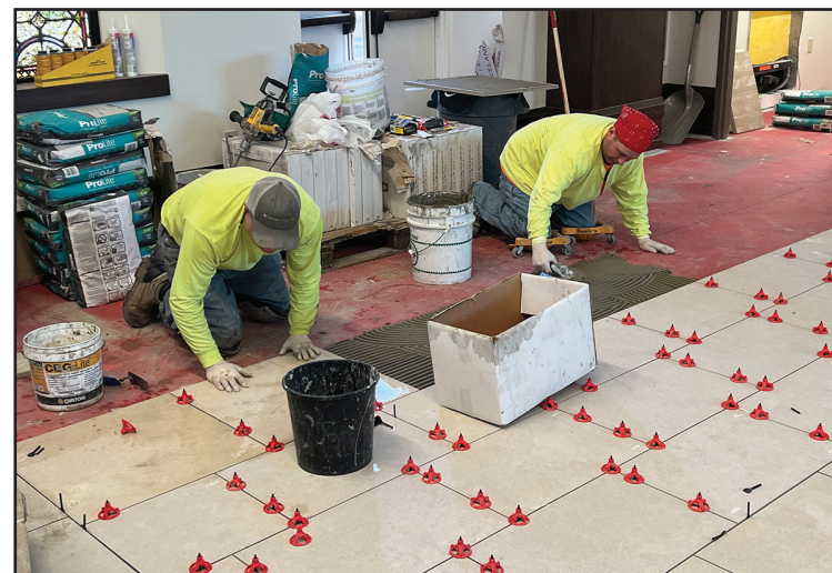
Workers place some of the last floor tiles in the main body of the new worship space for Most Holy Trinity Parish (Photos/Eric Deabill)
